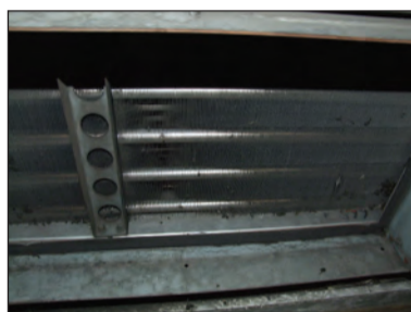
Dirty condenser coil.
