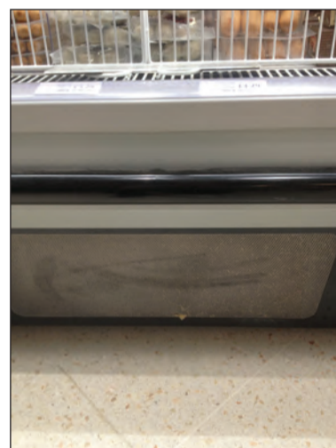
Refrigerated display cabinet intake with no air filter protection.
