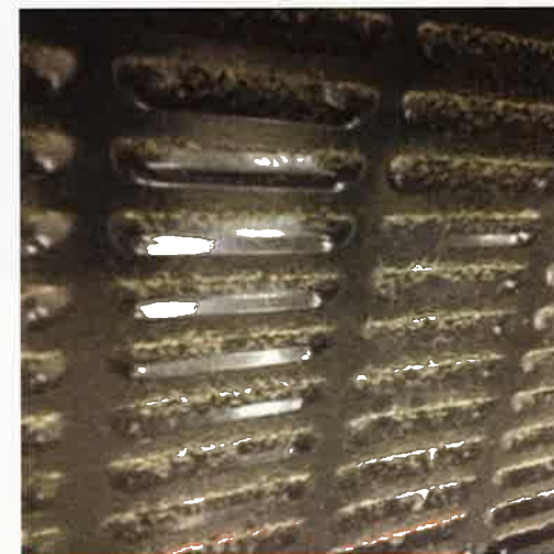
Dirt impacted air intake fins restrict airflow, leading to equipment failure.
