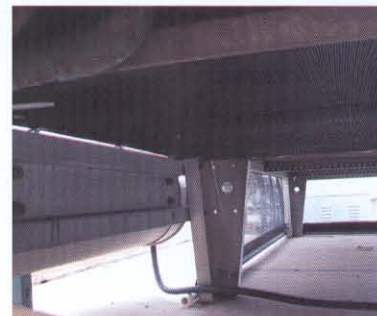
The air intake fins on a Liebert are located underneath the unit, making cleaning access extremely difficult.
